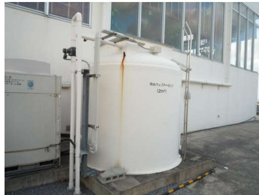
Buffer tank for rain water (2m 3 )
