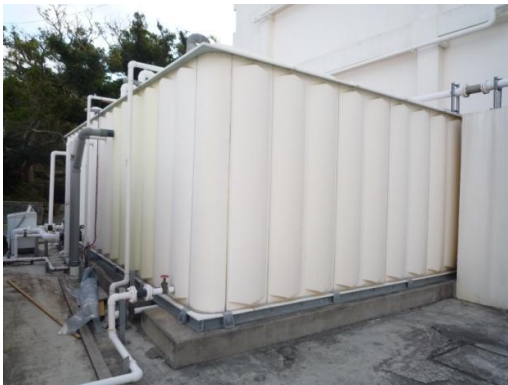
The receiving tank and the storage tank (50m 3 each)
