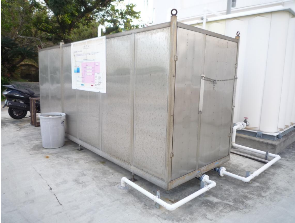
Waste water treatment equipment for reusing
